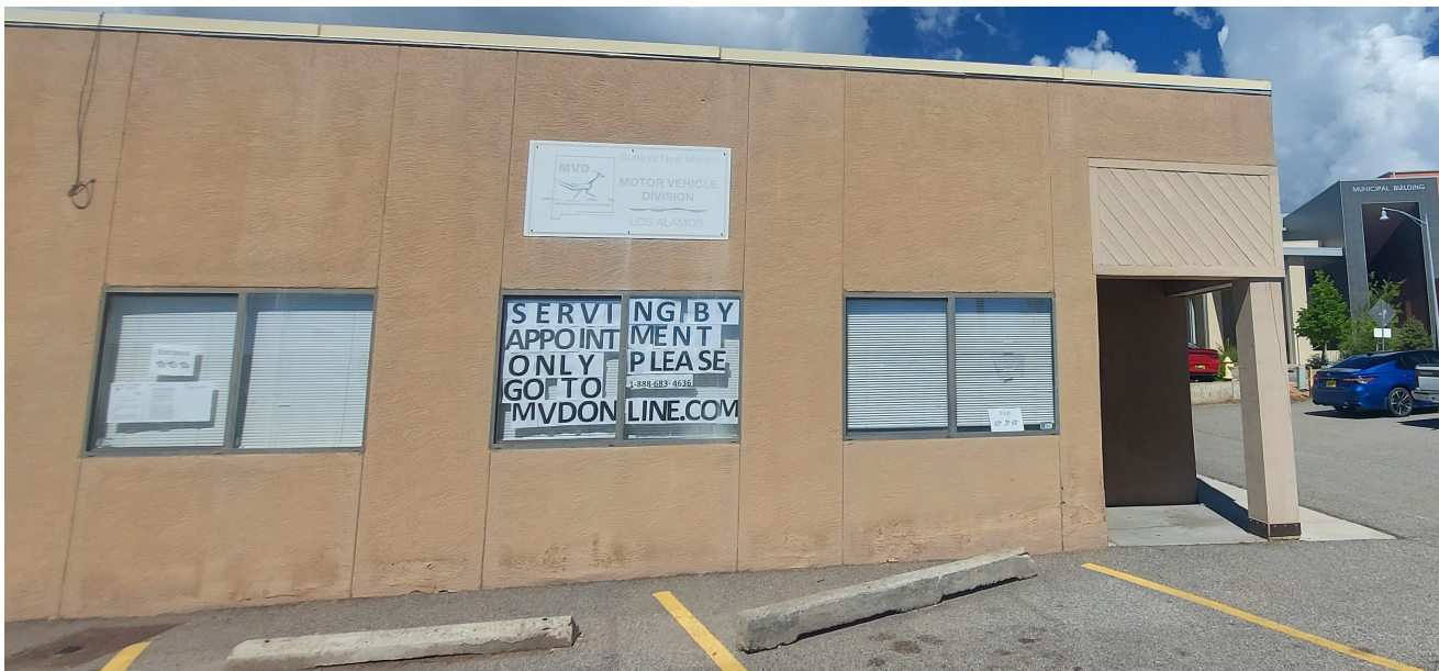
Figure 15. Deteriorating buildings are prevalent throughout the proposed MRA
