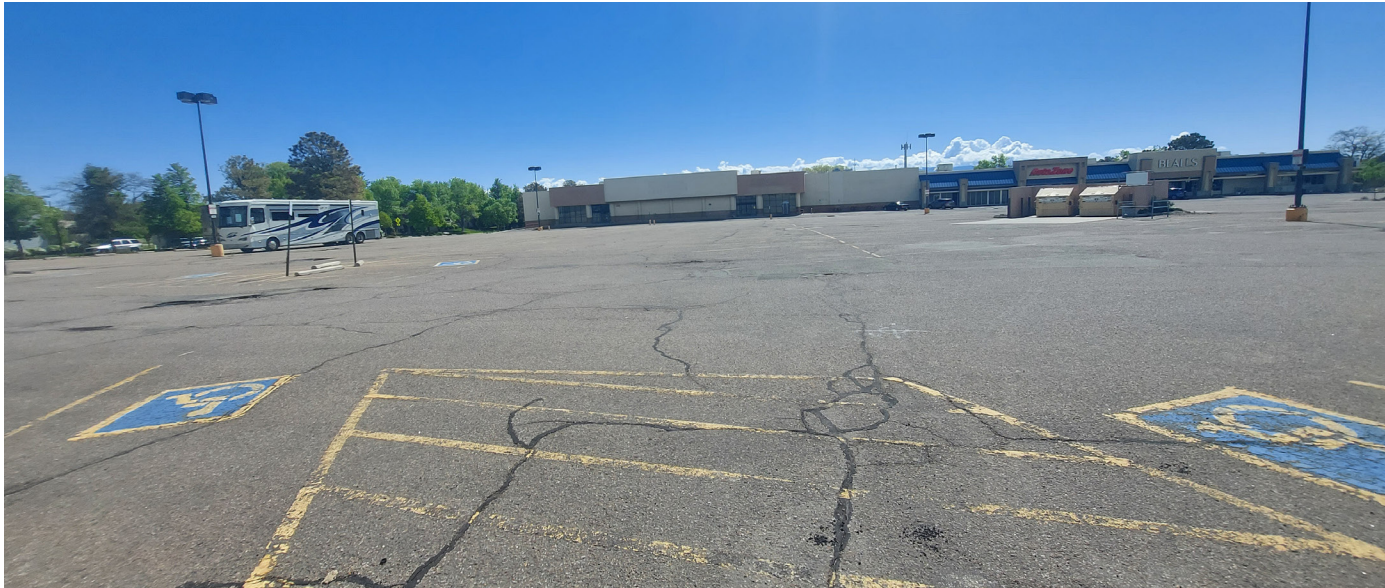
Figure 6. Extensive underutilized and deteriorating surface parking lots are present throughout the MRA
