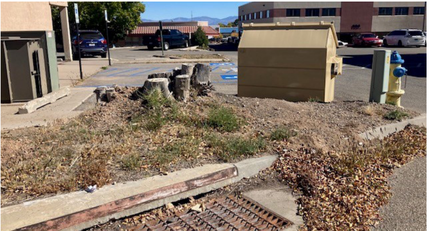
Figure 19. Unmaintained and deteriorating infrastructure are present throughout the proposed MRA
