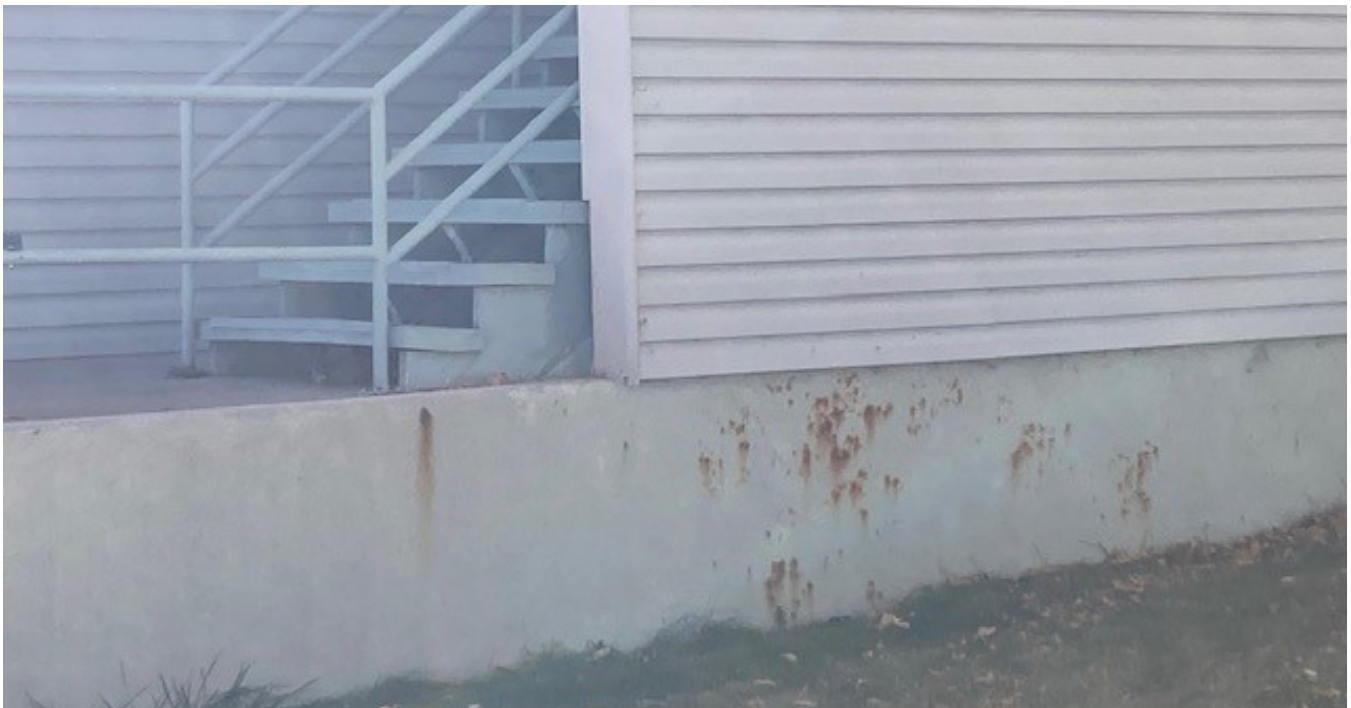
Figure 20. Multi-family housing facilities in need of renovation and repair
