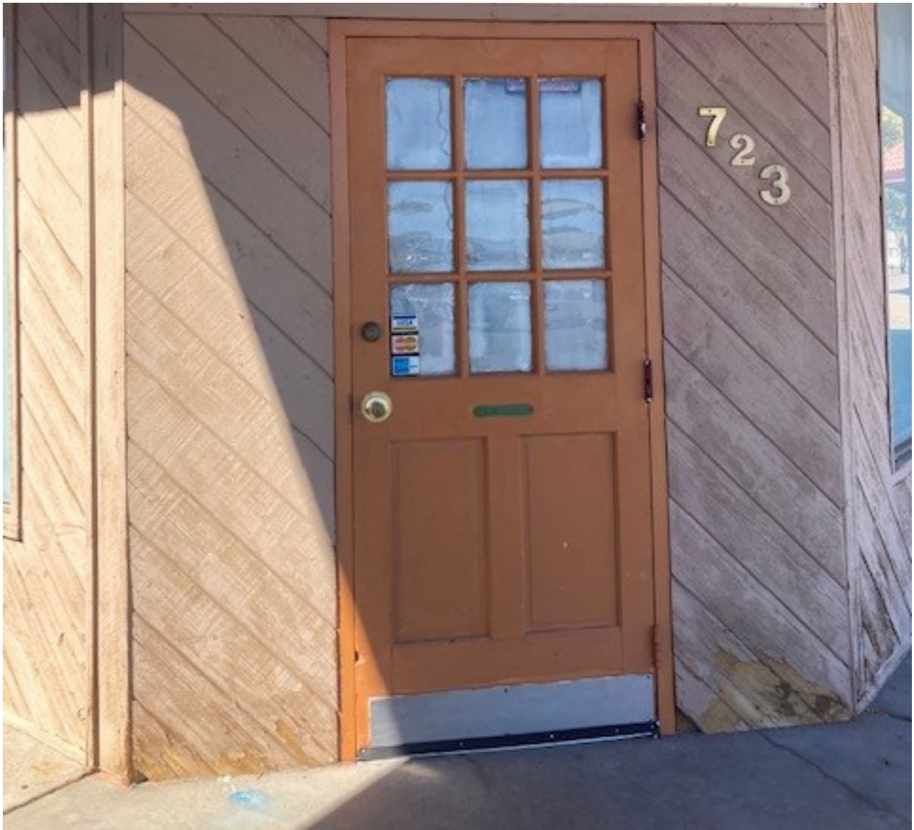
Figure 16. Deteriorating wood paneling is prevalent in the proposed MRA
