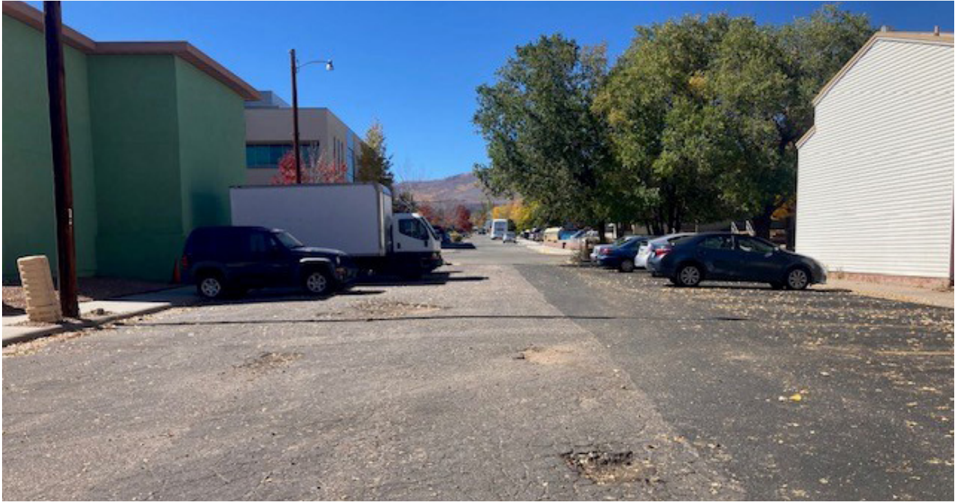
Figure 18. Deteriorating pavement on roadways and side streets is present throughout the proposed MRA
