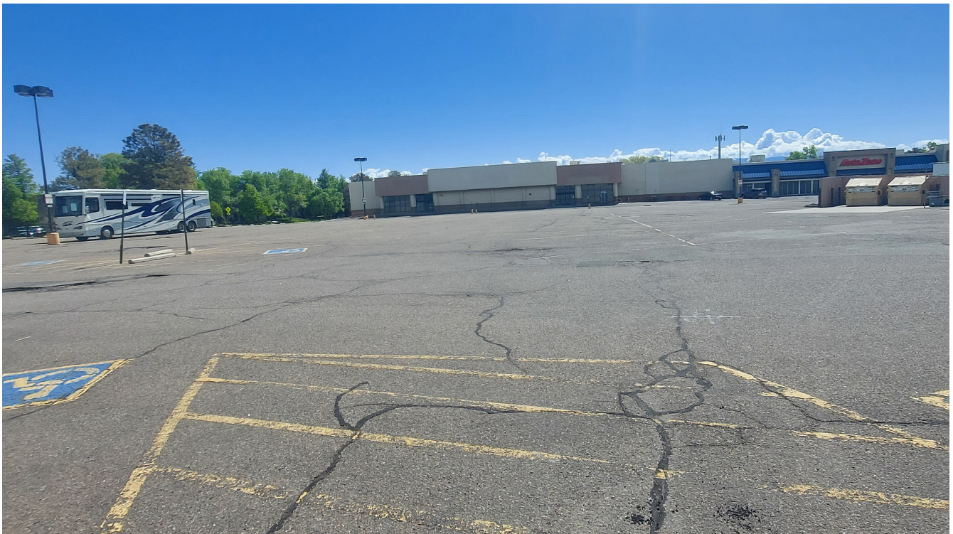
Figure 17. Deteriorating pavement on roadways and side streets is present throughout the proposed MRA
