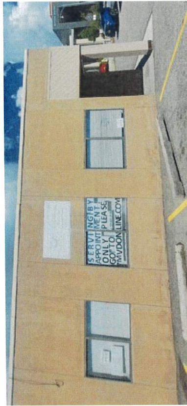
Figure 15. Deteriorating buildings are prevalent throughout the proposed MRA
