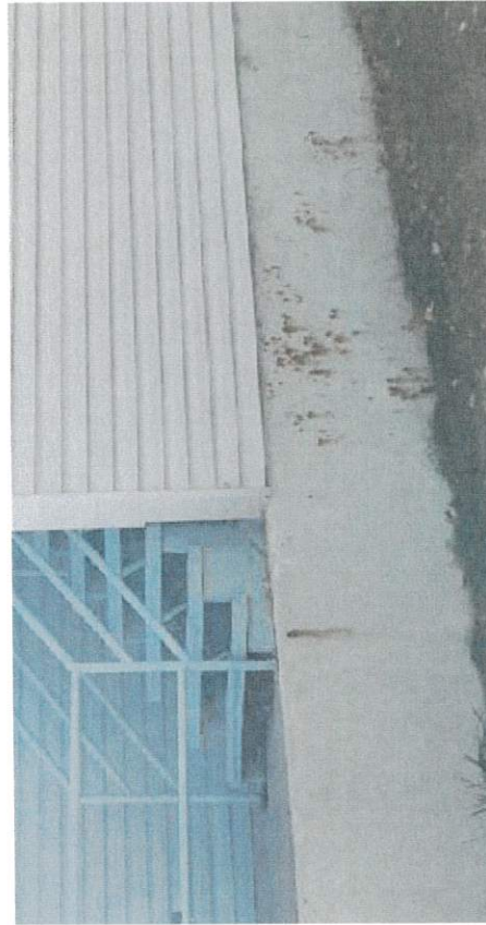
Figure 20. Multi-family housing facilities in need of renovation and repair
