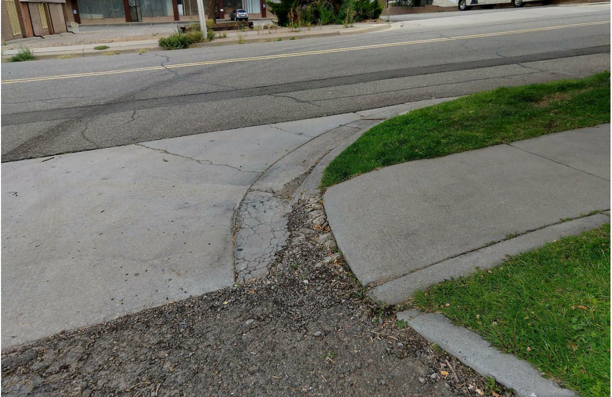
Figure 7. Degraded sidewalk conditions along the south edge of the Smith's Grocery property.
